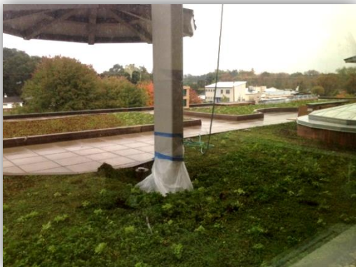
Green roof at Munson Cowell Family Cancer Center Photo courtesy of: The Watershed Center Grand Traverse Bay
